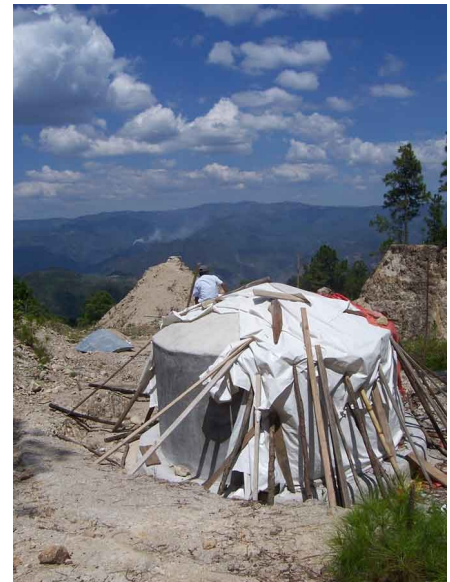
San Jose Centro water tank
