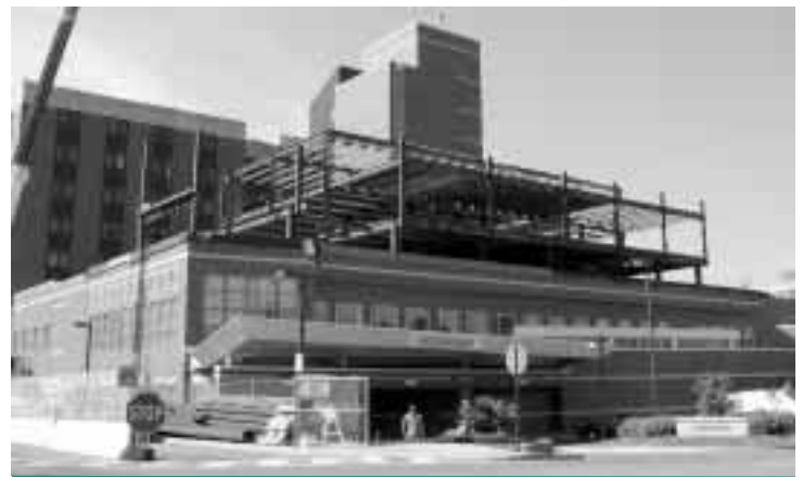
Construction of a new 22-bed Pediatric I.C.U. and Pediatric C.I.C.U. are under way.
