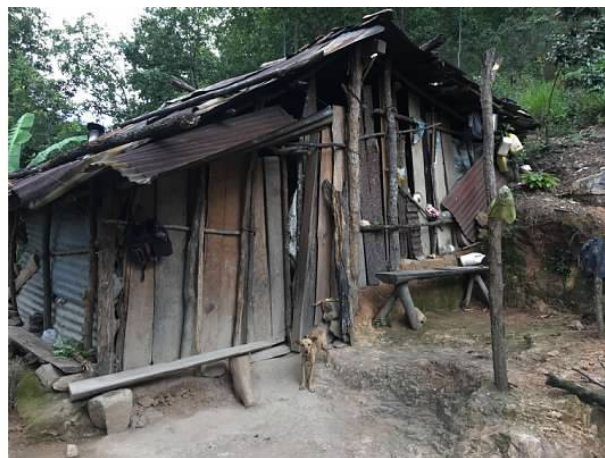
As this home demonstrates, much work remains to be done in San Jose
